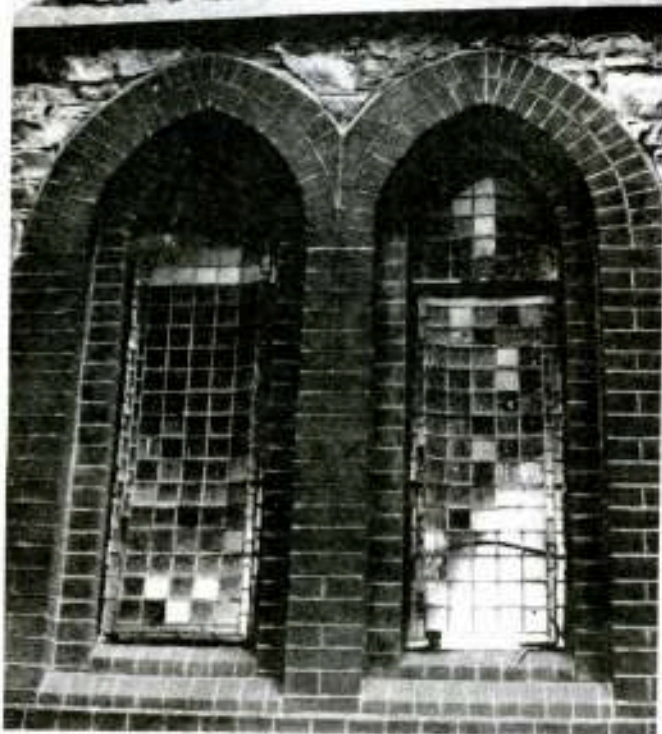
DETERIORATION OF WINDOWS (photo: Christ Church Cathedral Appeal)
