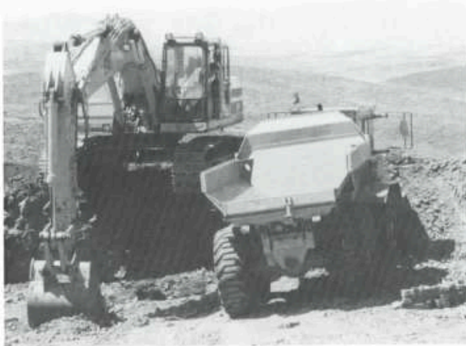
Earth moving equipment working on the new road from Port Howard to Chartres
